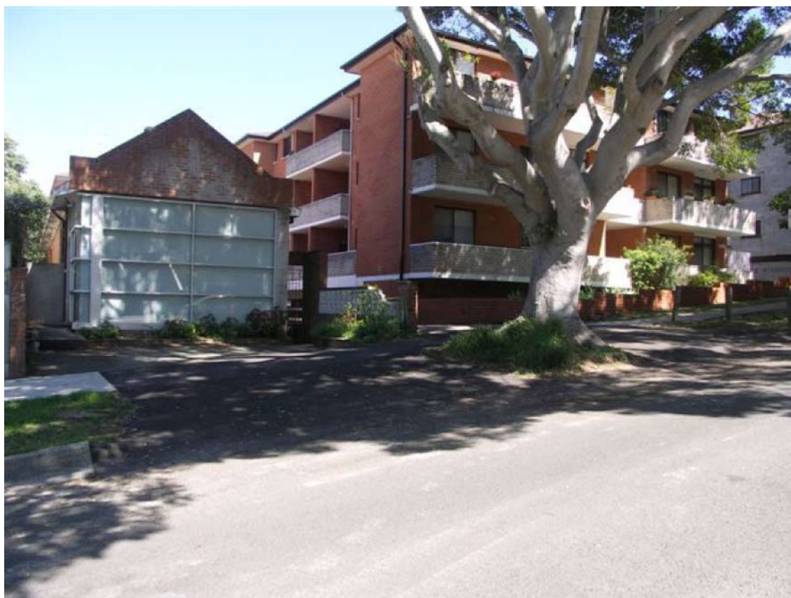
Image 10: Concrete kerb, gutter and footpath replaced with bitumen to minimise damage to tree roots
